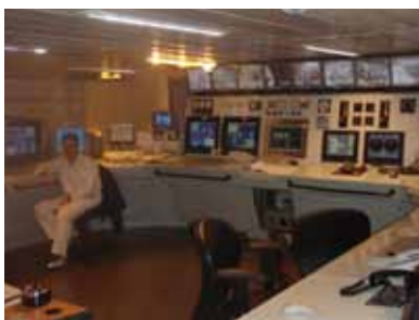
Engine control room
