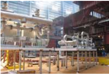
Components of the on-board Advanced Water Purification System (AWP)
