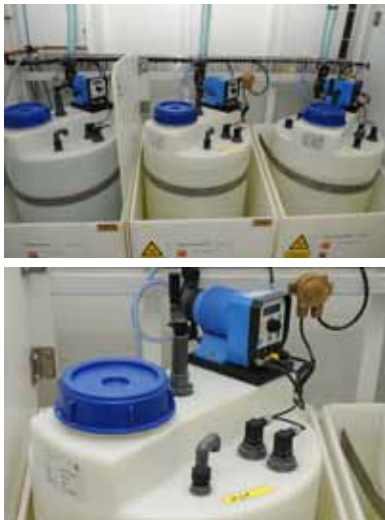
Potable Water Treatment
