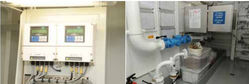
Left: Potable water analyzer, right: potable water bunkering
